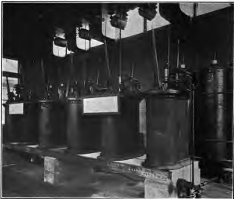
INTERIOR VIEW OF NORTH LAKE SUB-STATION SHOWING HIGH TENSION CIRCUIT BREAKERS AND WESTINGHOUSE ELECTROLYTIC LIGHTNING ARRESTERS
